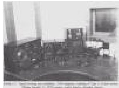
Receiving radio equipment of the 1914 era. The caption reads: "Typical receiving room installation. 1914 equipment consisting of Type A (Cohen) receiver, Wireless Specialty Co. (IP75) receiver, crystal detector, ultraudion detector."
